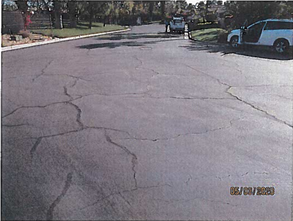
PHOTO 8 Continuous slight to severe block cracking is depicted in this photo.
