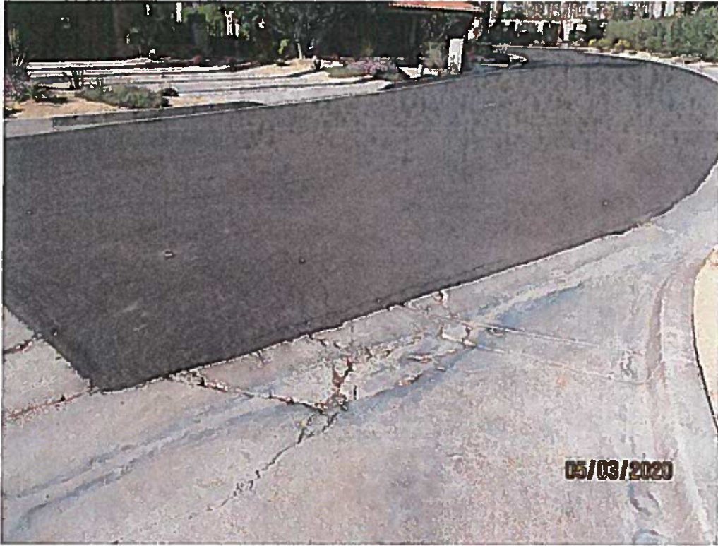
PHOTO 7 Typical PCC repair needed is depicted in this photo.
